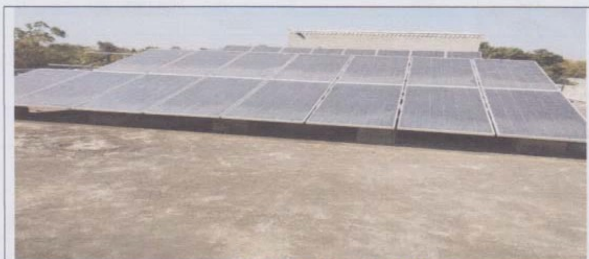
Fig 4: Solar panels of 10 kw
